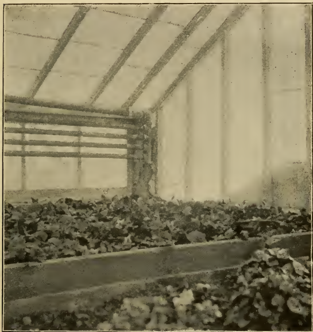
20.—Interior of house, showing method of connecting flow pipe with four returns
